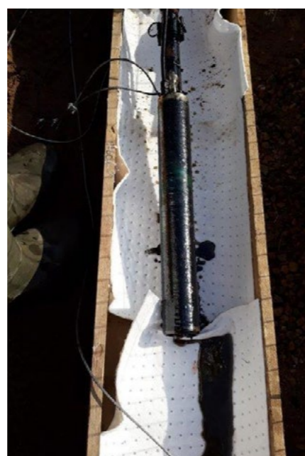
Figure A6.11: Solar-powered coal tar recovery system at Howdon Lane, Newcastle
