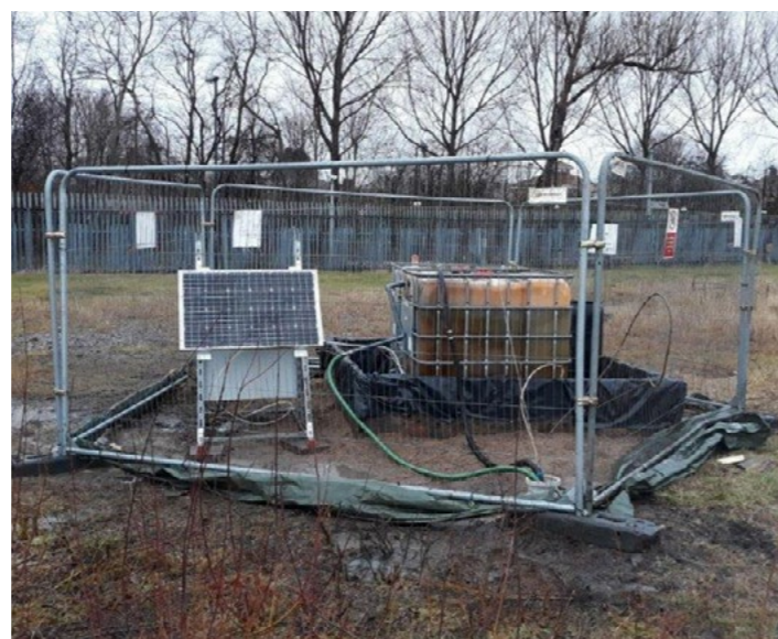
Figure A6.10: Solar-powered coal tar recovery system at Howdon Lane, Newcastle
