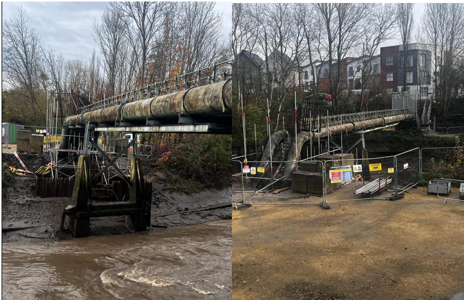
Figure 2 Team Street overcrossings showing ineffective pipe support and temporary supports during the construction phase (LEFT: facing West; RIGHT: facing East)
