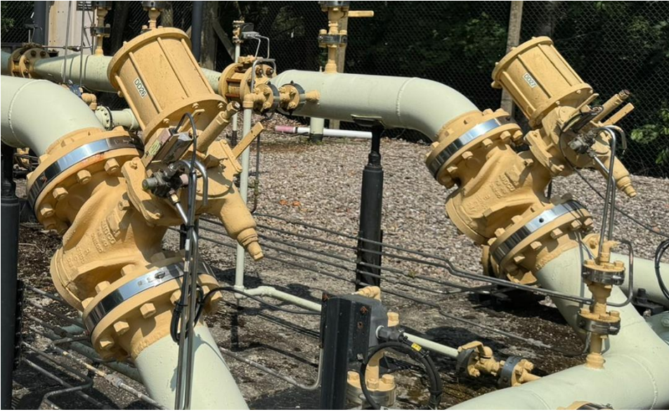
Figure 2 photograph showing lineguard system
