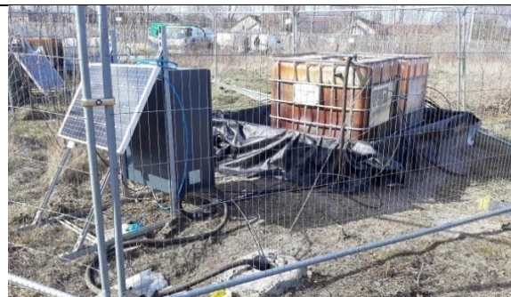
Figure 1 - Solar power coal tar recovery system at Howdon Lane, Newcastle.
