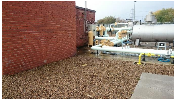
Congested works area – accessible portion of tank under gravel cover adjacent to live gas infrastructure
