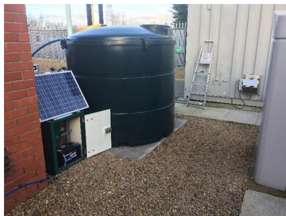
Pumping equipment installed around gas infrastructure
